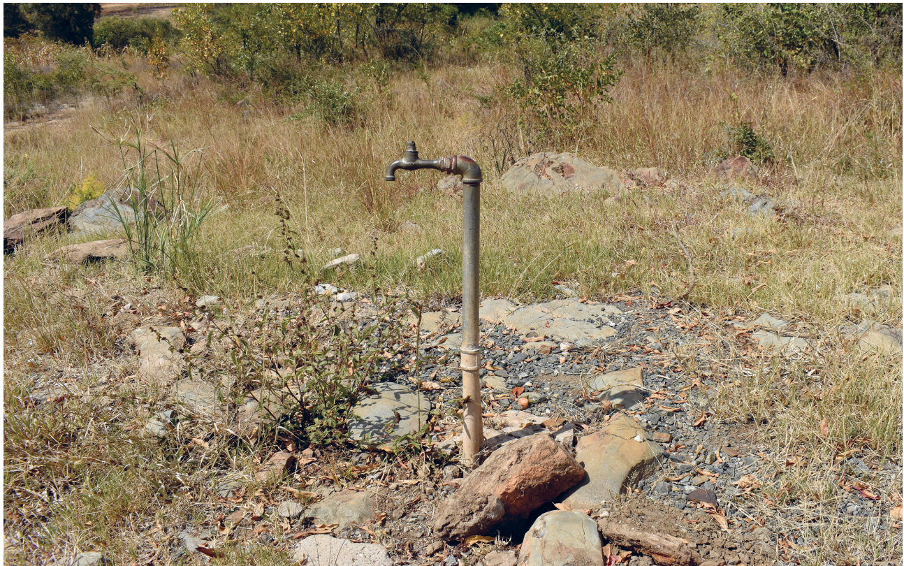
Destroyed tap next to a cistern in Bikita.
